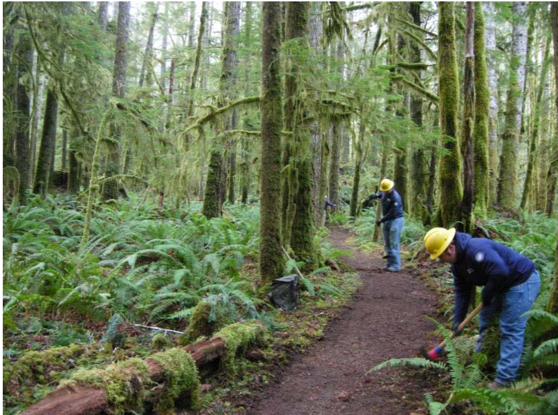
Building an accessible trail near the Duckabush River in Olympic National Forest
