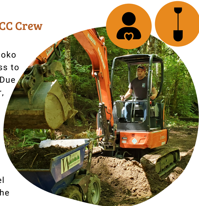
Volunteer Matthew Berberich runs the excavator as our WCC crew hauls out the culvert and fill from the fish barrier.
